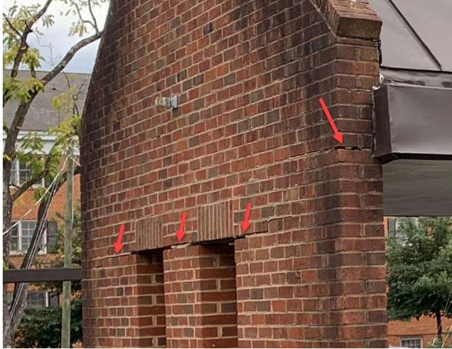
Image 4. Visual disrepair in brick joints
