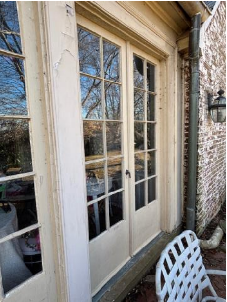
ENCLOSED PATIO - DOOR DAMAGE
