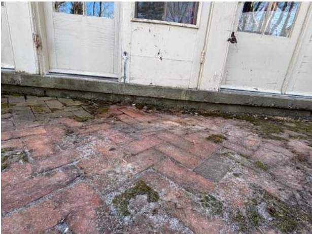
ENCLOSED PATIO - DOOR DAMAGE
