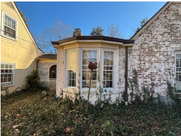
BAY WINDOW - ROT/DAMAGE
