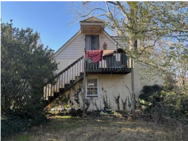
GARAGE - RIGHT SIDE VIEW (FROM DRIVEWAY)
