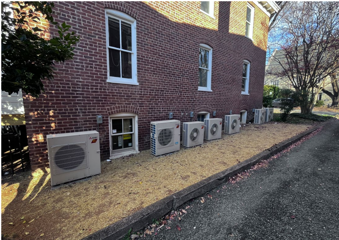
Mechanical units at side yard, November 2024
