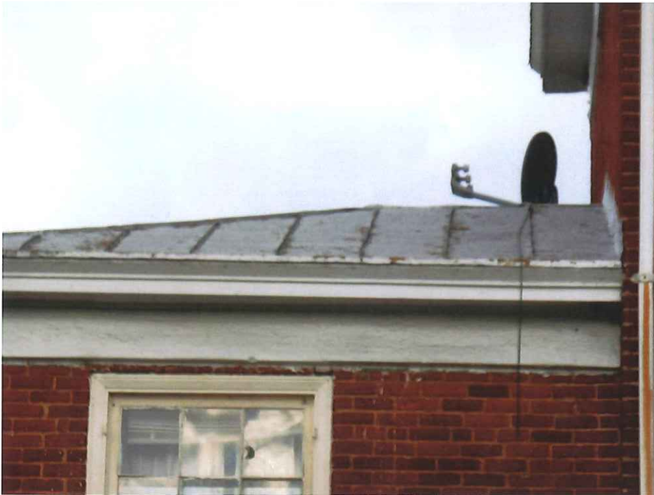
Investigate condition of gutters and repair any rusted sections. Scrape, prime and repaint existing standing seam roof with silver roof paint matching existing.
