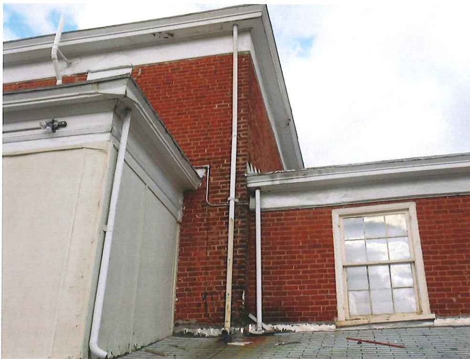
Rust-through holes in downspouts.
