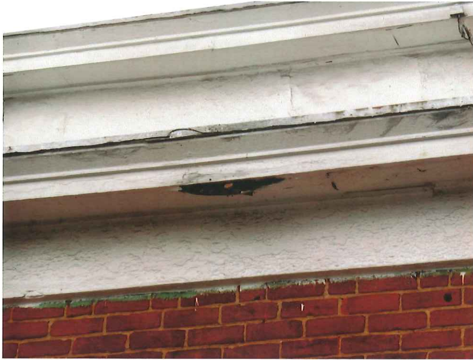
Repair small sections of water damaged wood soffits.
