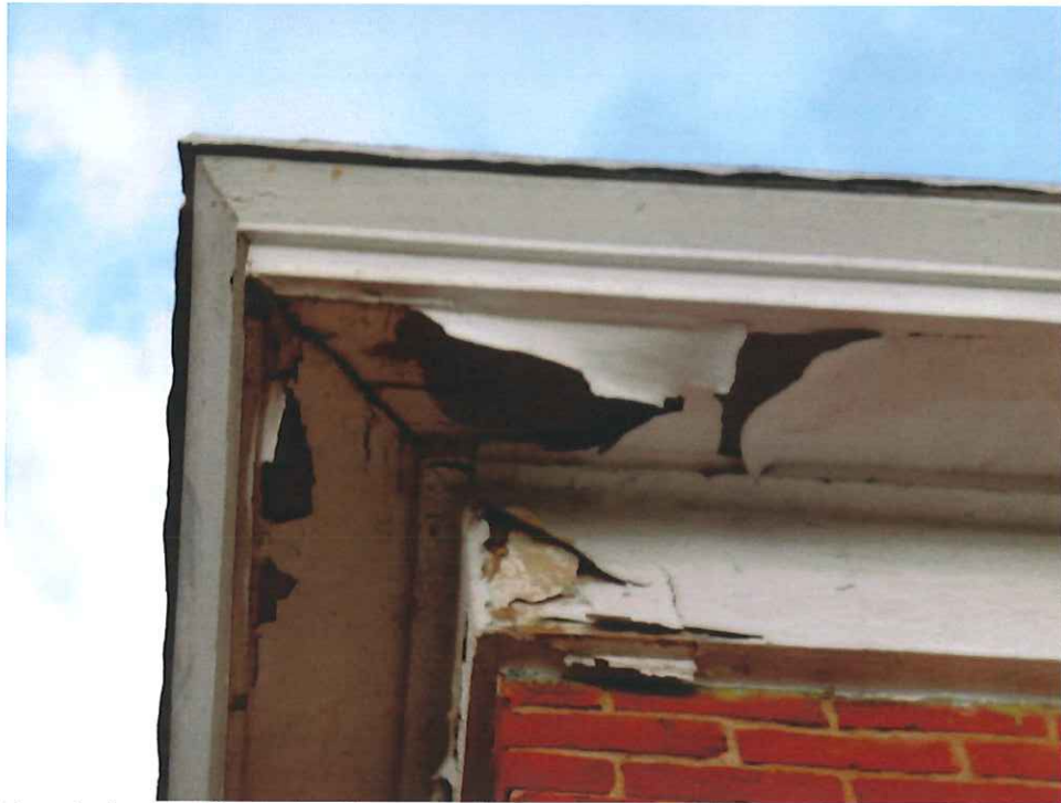
Repair damaged wood soffit at rear corner.
