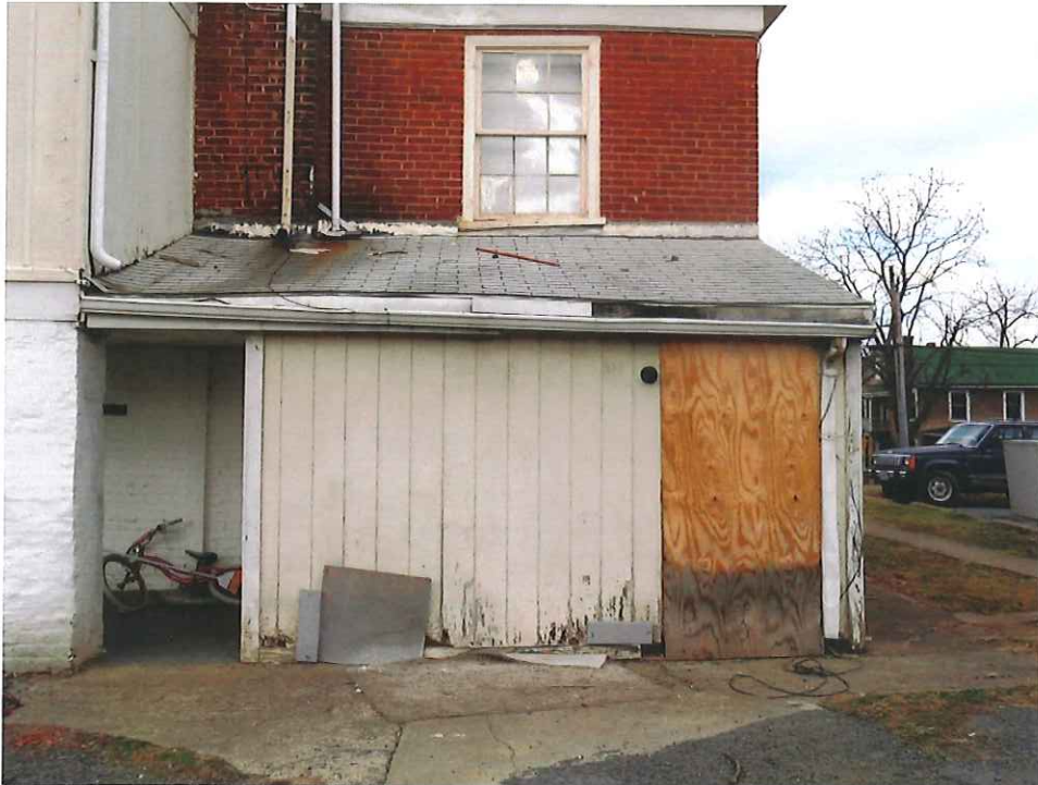
Rear addition to be re-sided. Provide concealed flashing behind siding and seal at slab level, to keep water from seeping in under wall. Replace damaged sill and framing inside as required.
