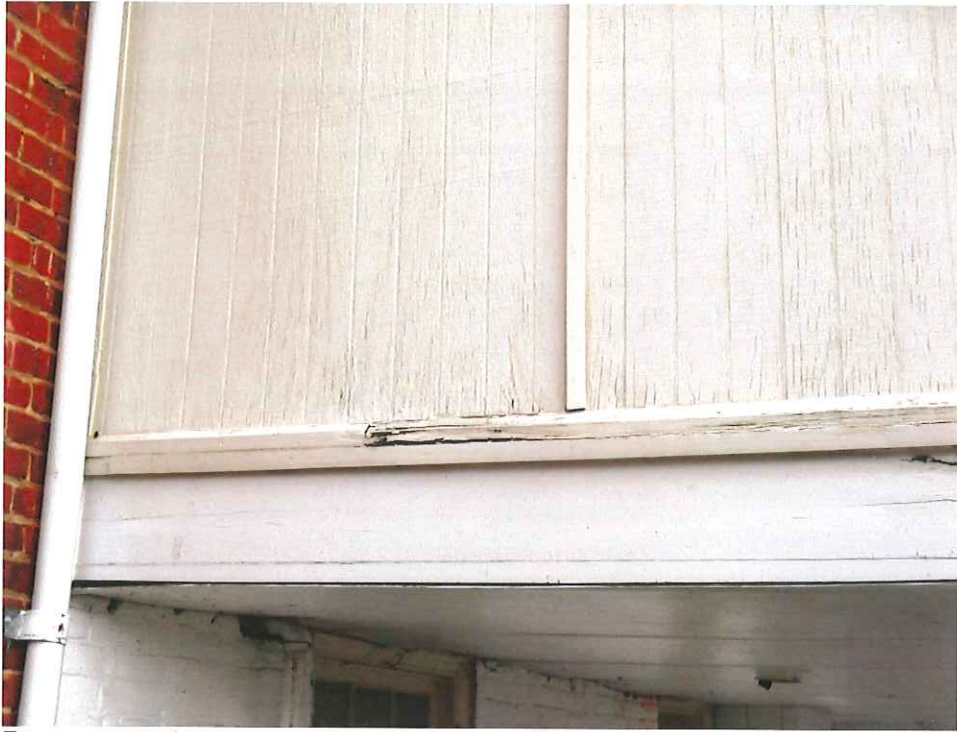
Remove rotted wood trim. Lap existing horizontal trim with concealed "Z" flashing run under new Hardiplank siding.
