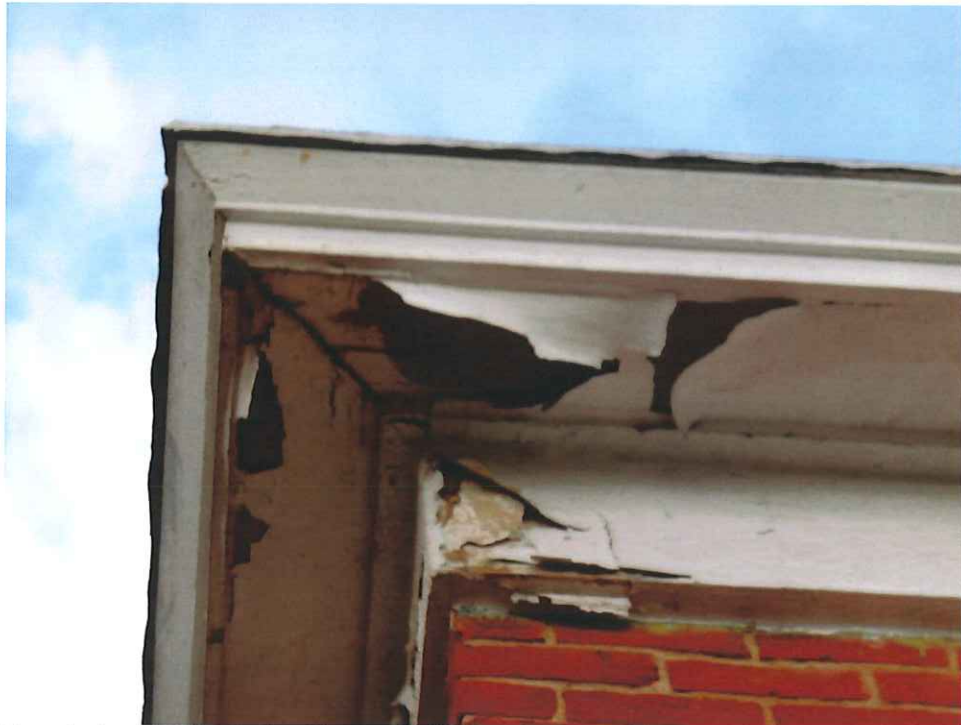
Repair damaged wood soffit at rear corner.
