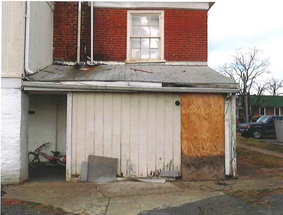
Rear addition to be re-sided. Provide concealed flashing behind siding and seal at slab level, to keep water from seeping in under wall. Replace damaged sill and framing inside as required.
