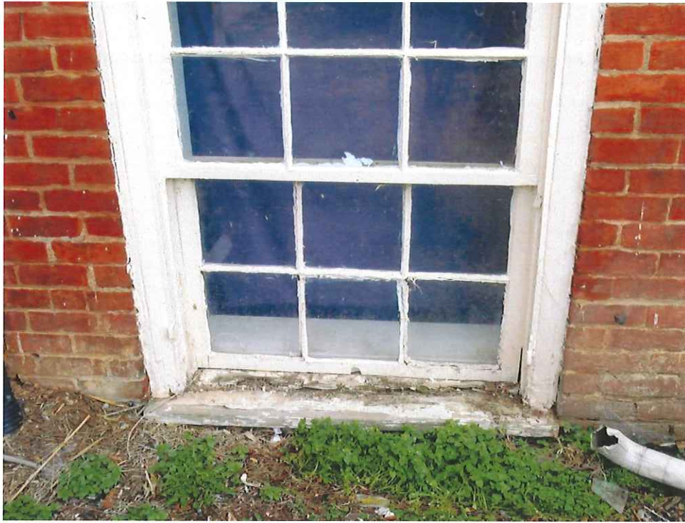
Basement window sills have wood rot. Lower grade soil to provide for drainage away from the building and replace damaged wood.
