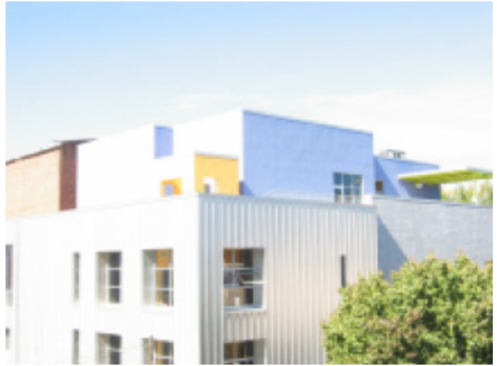
Rooftop screening of mechanical equipment can provide an opportunity to continue design elements at roof level.
