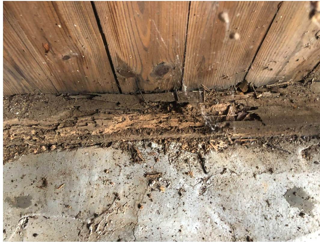
TERMITE DAMAGE AT SILL PLATE
