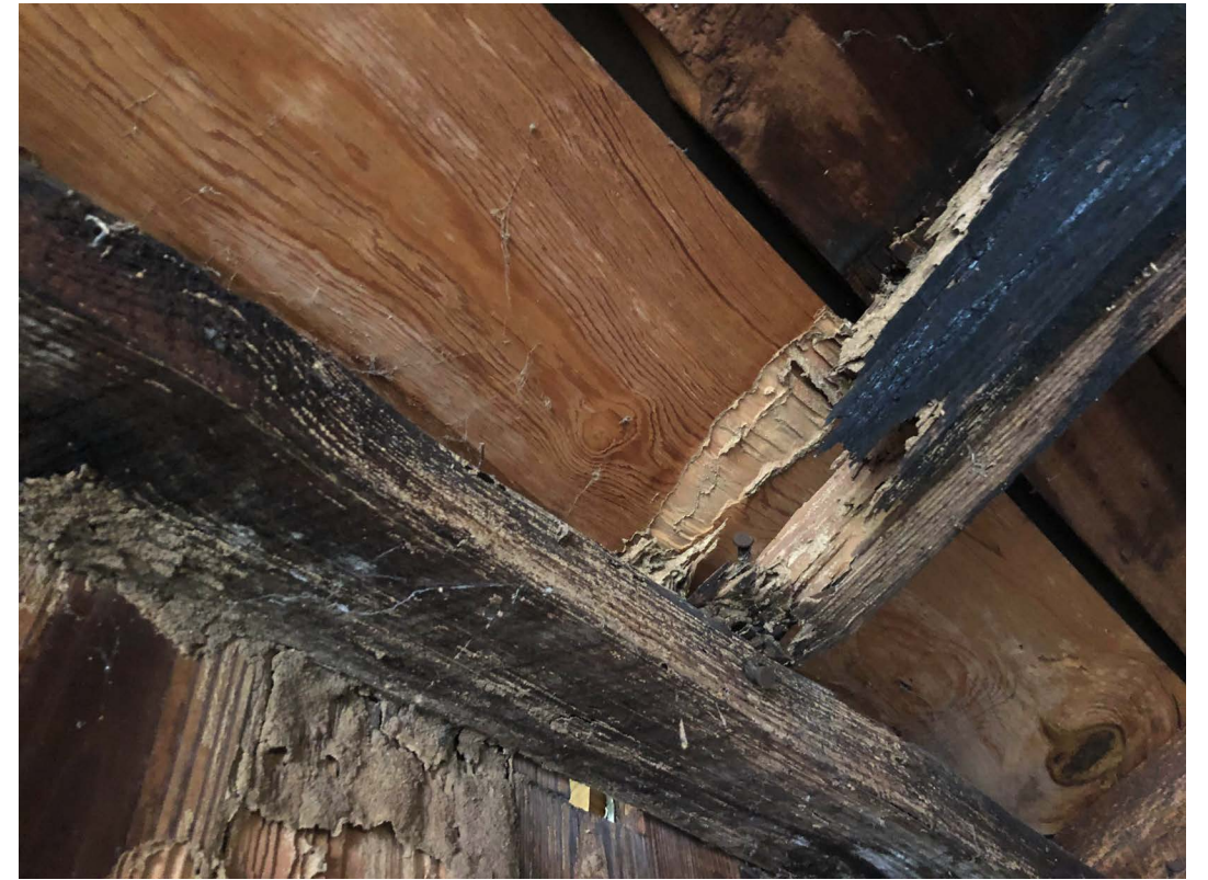
TERMITE DAMAGE AT EXISTING RAFTERS
