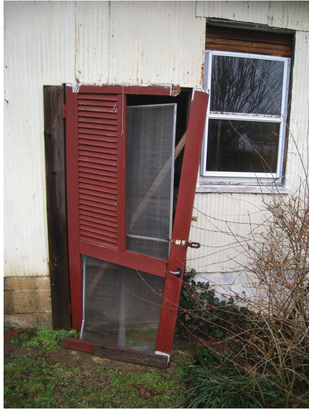
DAMAGE TO EXISTING DOOR
