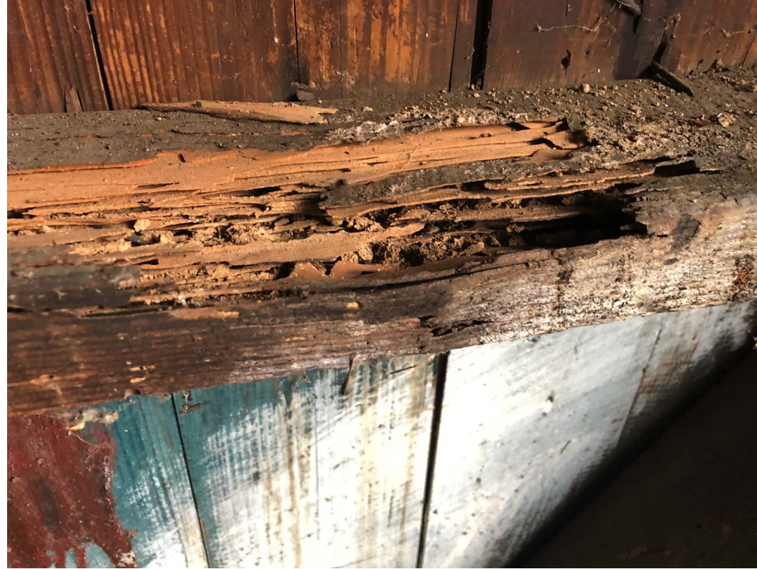
TERMITE DAMAGE AT WALL FRAMING
