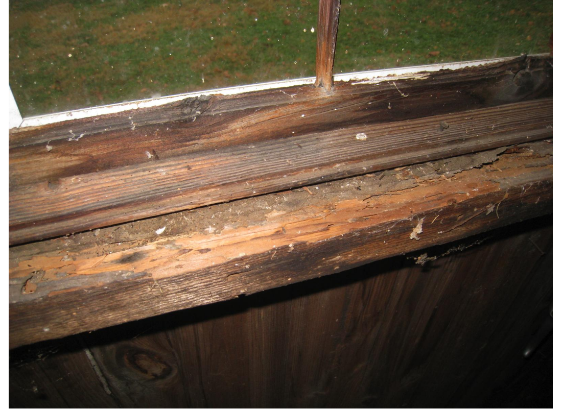
TERMITE DAMAGE AT WINDOW SILL
