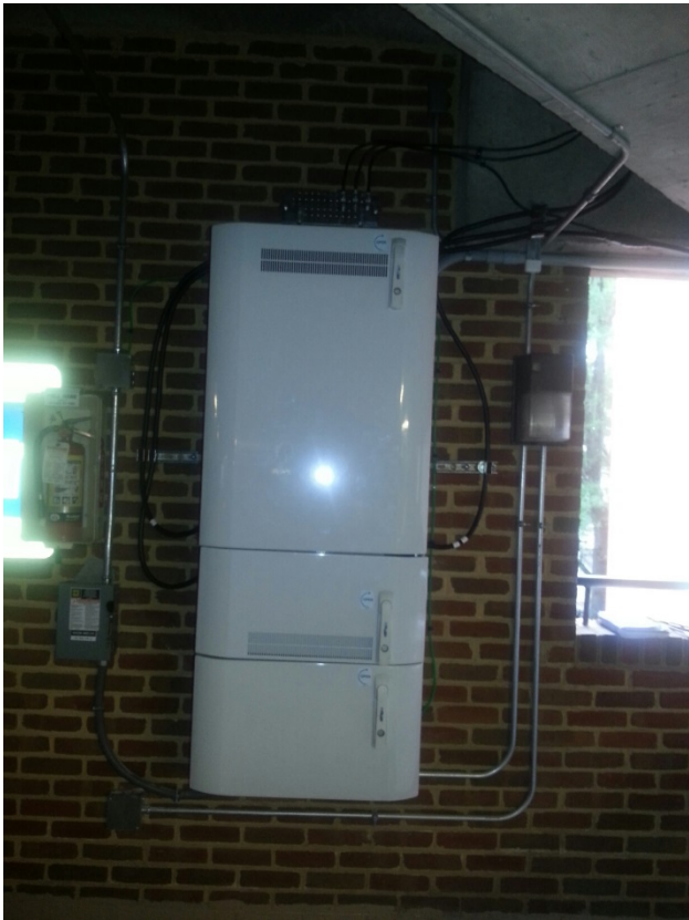
Equipment Box Mounted inside Building Near Elevator Shaft
