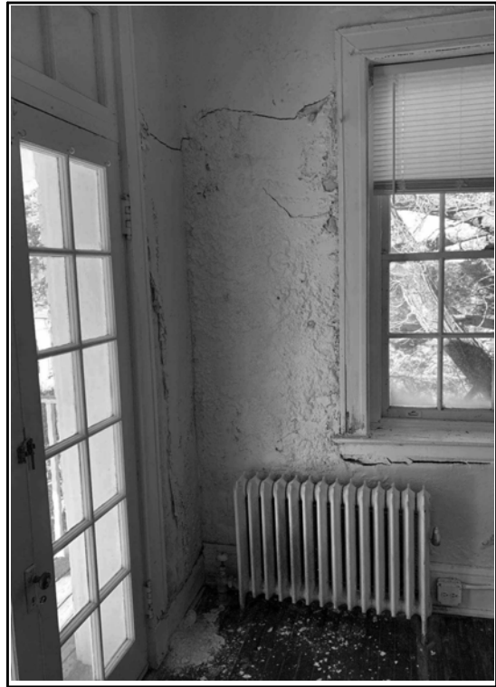
DETERIORATED PLASTER (TYPICAL THROUGHOUT THE BUILDING)
